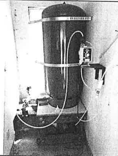
West Well Chlorine Hook Up Facilities
