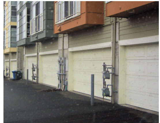
Figure 3-24. Exposed utility meters like this will not be allowed.
