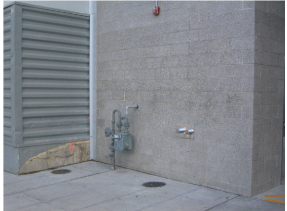
Figure 5-14. Avoid exposed utility meters along the sidewalk, like this.
