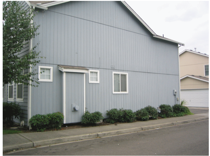
Figure 4-14. T-111 siding is prohibited.
