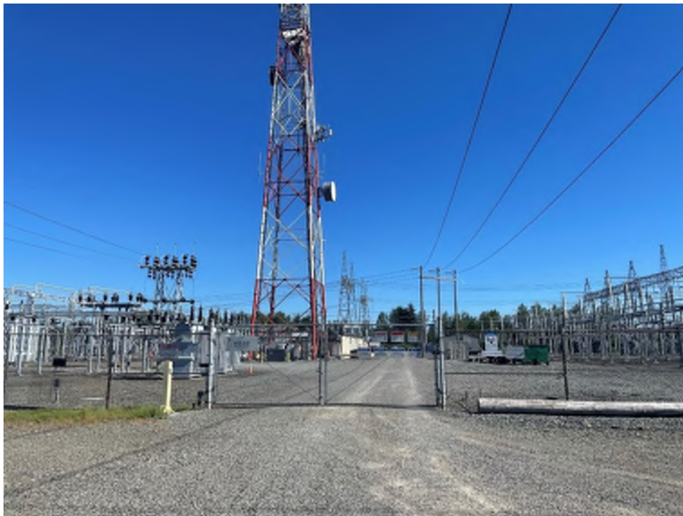
Photo 10 View of the east-adjointing White River Substation (2120 Lakeland Hills Way), located east of Parcel B, from the east-adjointing property facing north.
