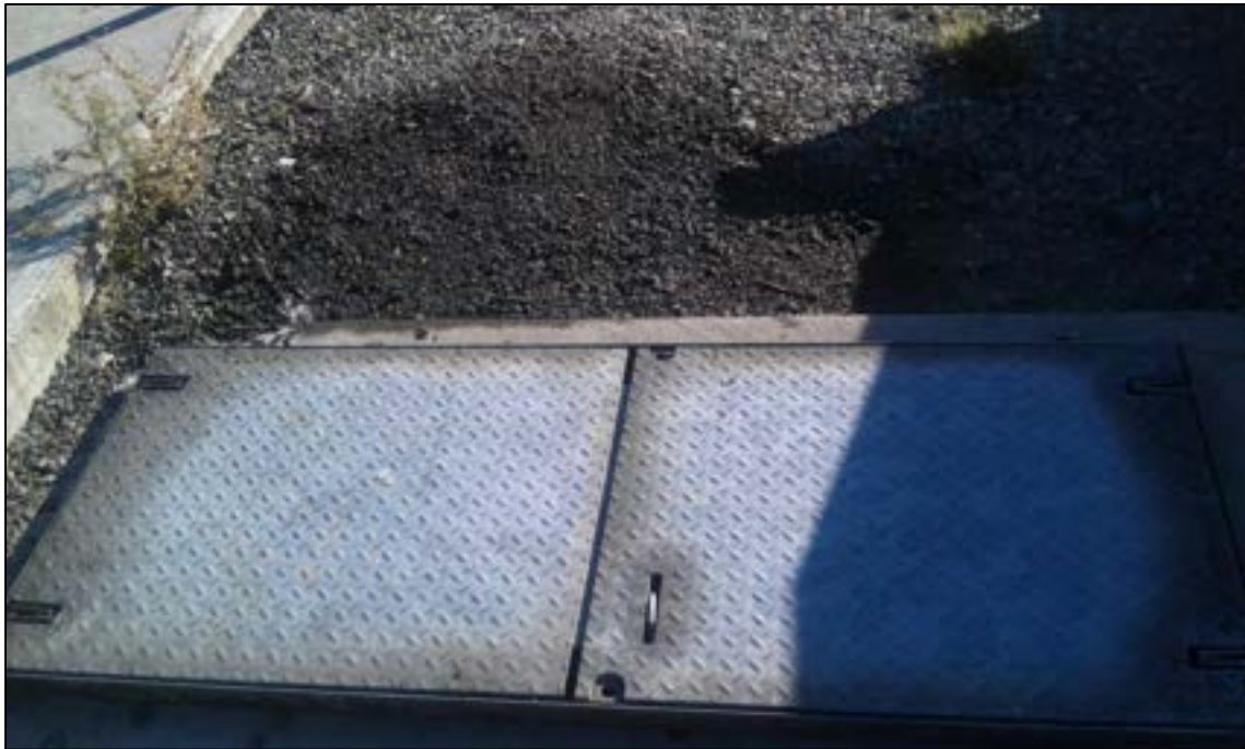
Photograph 23: Staining observed at punch auger truck oil-water separator.
