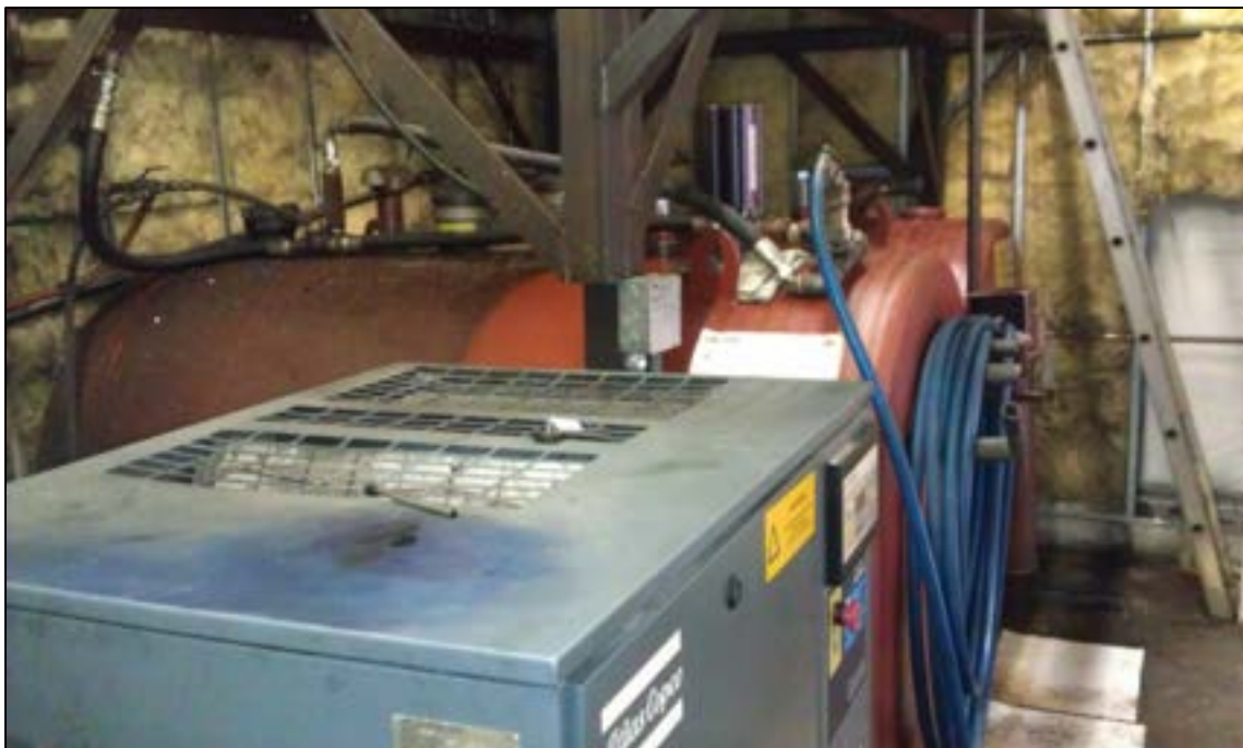
Photograph 38: Lower ASTs in Building B oil storage room.
