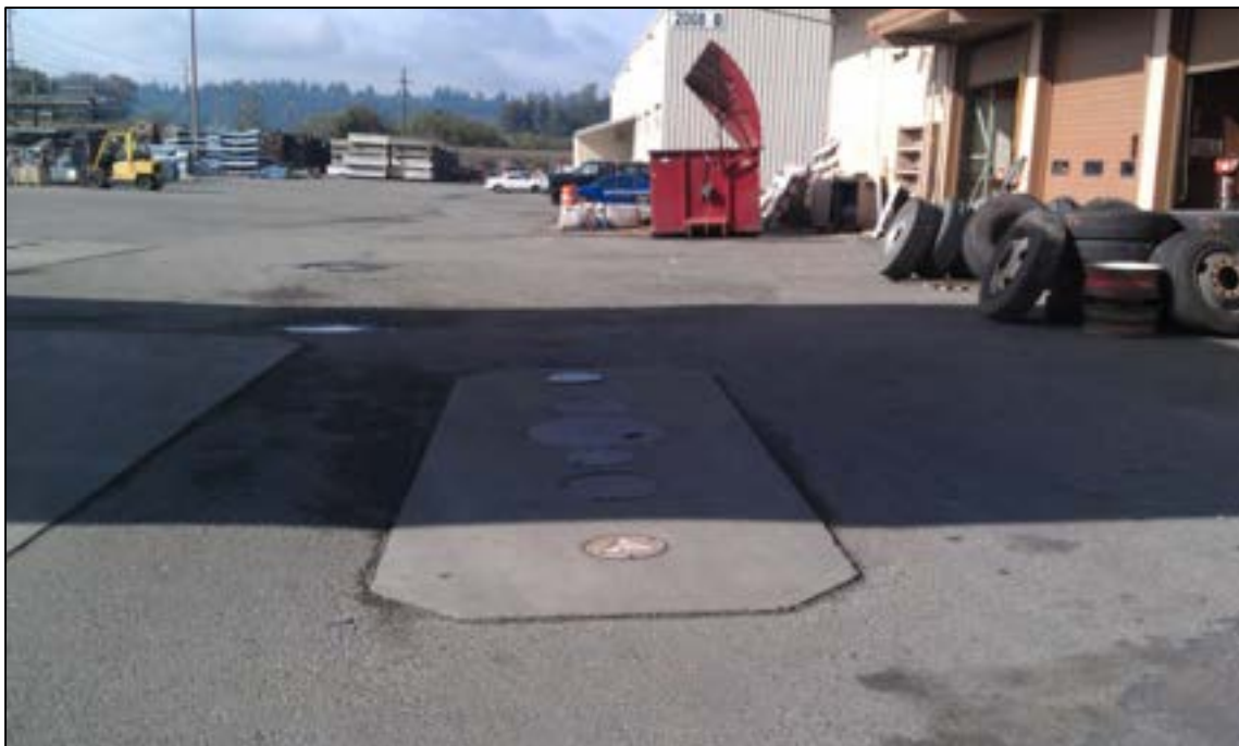
Photograph 24: 1,000-gallon waste oil UST north of fuel canopy.
