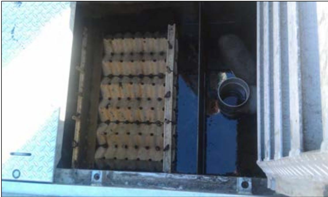
Photograph 25: Oil-water separator west of UST nest.
