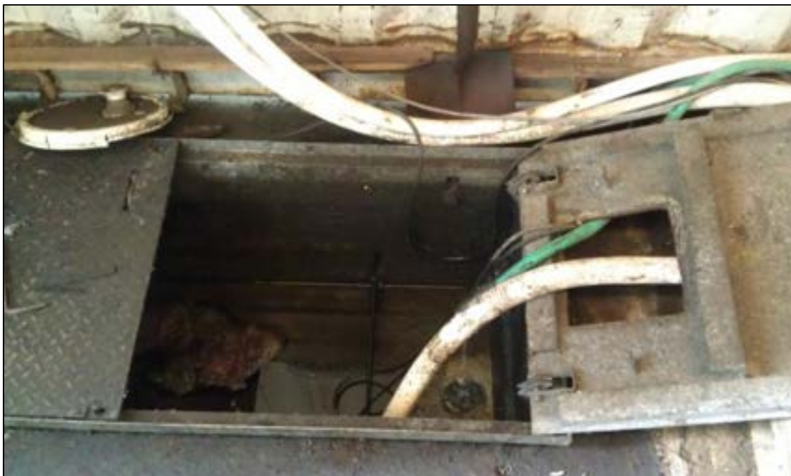
Photograph 26: Oil-water separator at washbay.
