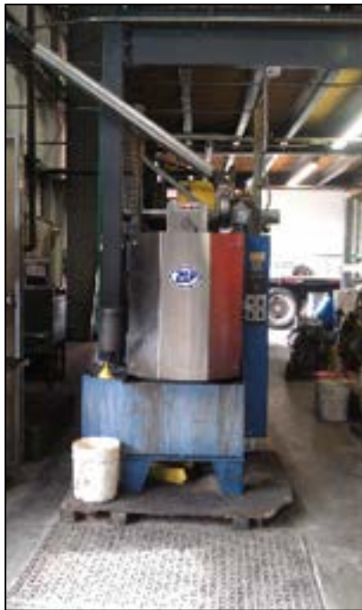
Photograph 36: Hot water/steam parts washer in Building B.
