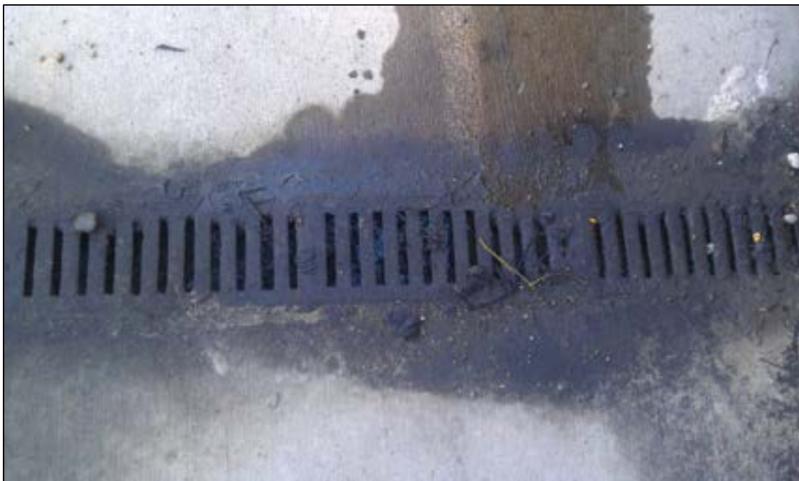
Photograph 22: Significant staining was observed near the punch auger truck trench drain.
