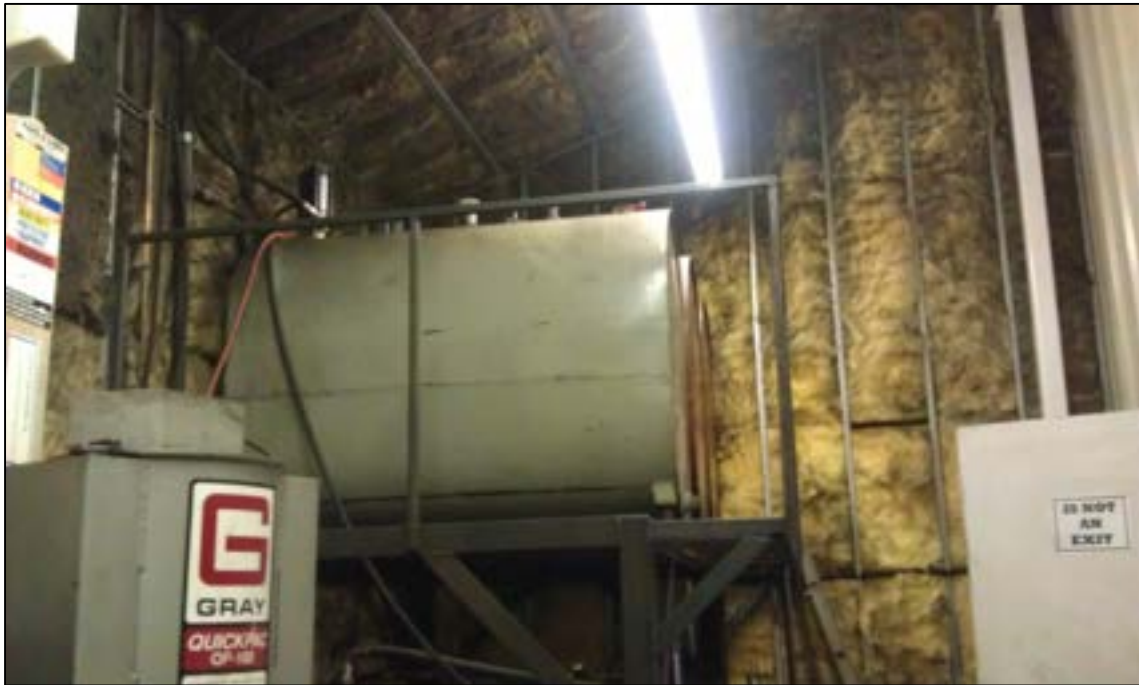
Photograph 37: Upper ASTs in Building B oil storage room.
