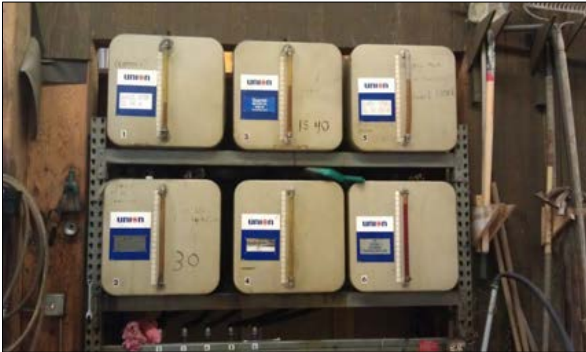
Photograph 29: Oil storage at work pit in Building A.
