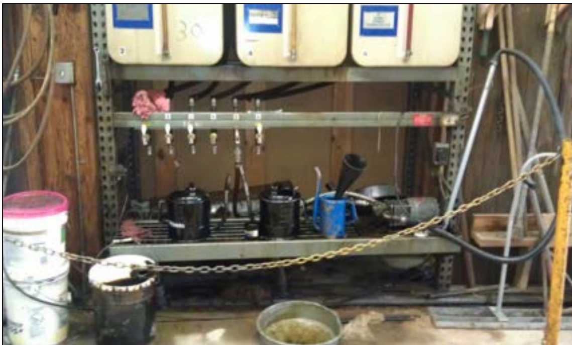
Photograph 30: Drip tray beneath oil storage at work pit.
