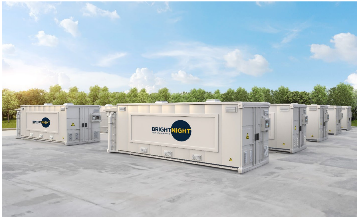
Photo 1. Example of BESS module energy units in rows
