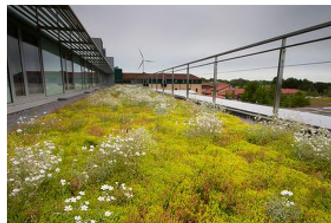
EXTENSIVE GREEN ROOF, SEDUM AND WILDFLOWER MIX
